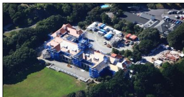
Government House covered in scaffolding while restoration and conservation work is undertaken, March 2010.
